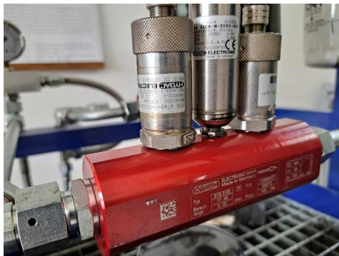
Obr. 7 Združené meracie zariadenie HYDAC so senzormi na meranie (zľava) tlaku, prietoku a teploty (from left) Pressure gauge, flow meter and thermometer sensors as combined measurement device HYDAC
